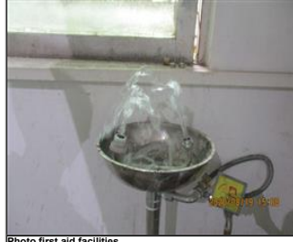
Photo first aid facilities Eye washing facility.JPG
