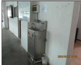
Photo of the sanitary facilities Potable water.JPG
