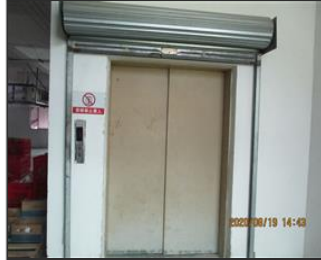
Photo of the inside of the main production hall Elevator.JPG
