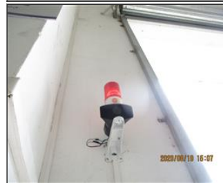
Photo of fire safety equipment Fire alarm flashing when tested.JPG
