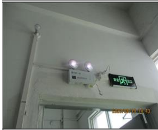
Photo of fire safety equipment Emergency light.JPG
