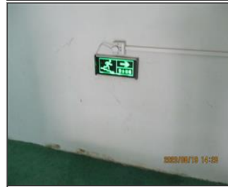
Photo of fire safety equipment Evacuation sign.JPG
